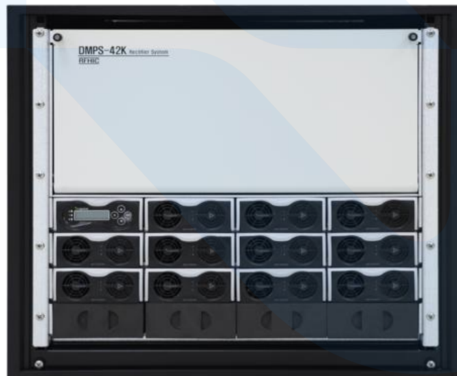
Figure 2: Power Supply Unit Front View
